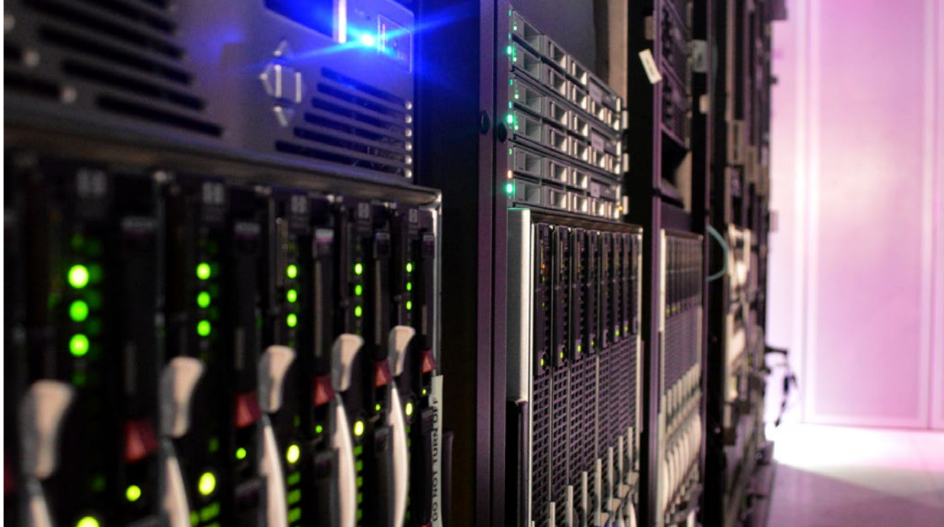
EMBL-EBI data centre in Hinxton, UK
