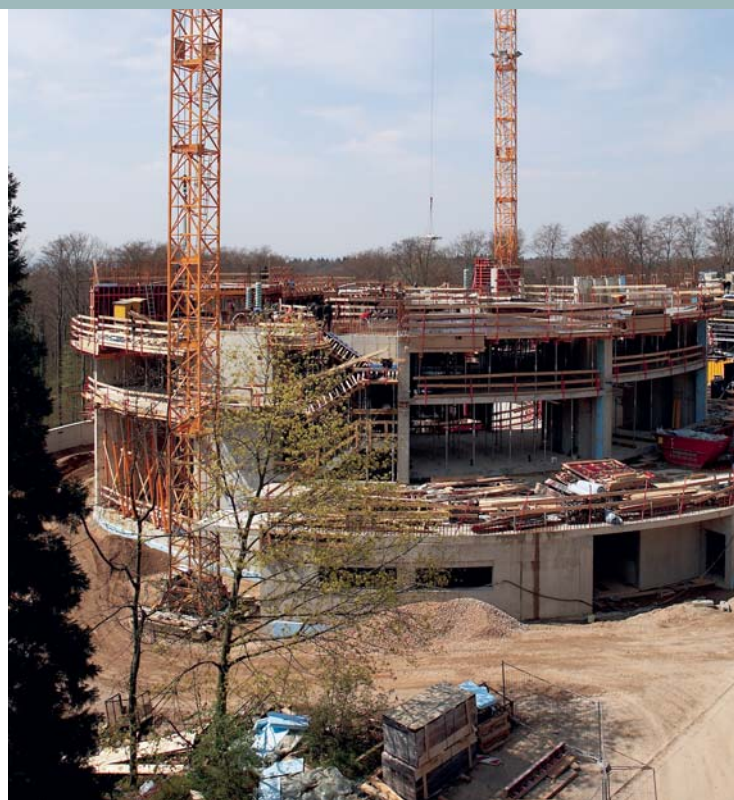
The helical architecture of the Advanced Training Centre on the Heidelberg campus is already recognisable.
